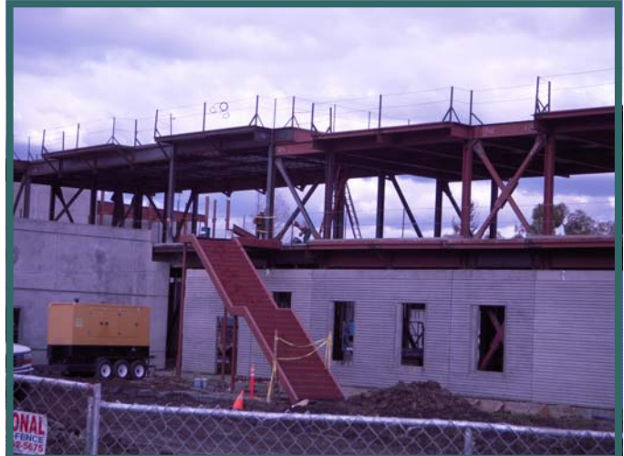
Photo taken in April 2009 by Isabel Braunstein during construction of the CSSC (Building 700)
